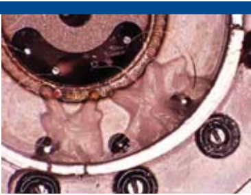
Naval Surface Warfare Center (NSWC): Defective hardware found and replaced.
